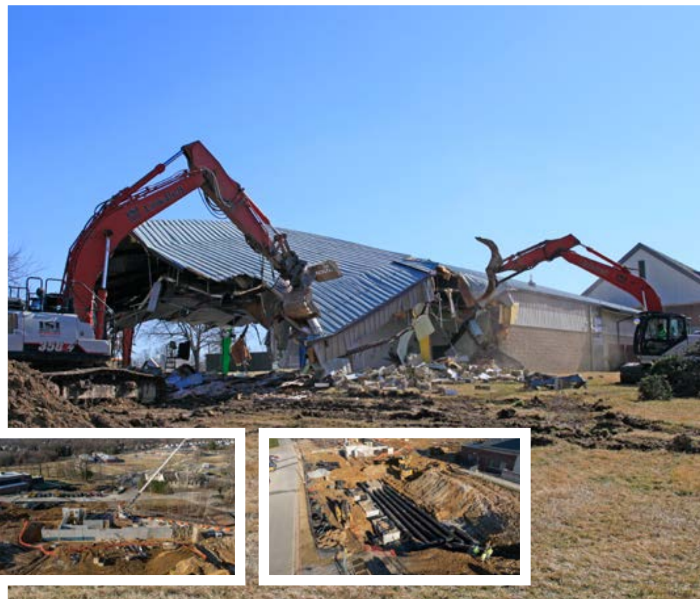
These images capture the transition from the demolition of the old pool to the construction of the new facility, reflecting MSB's history and its commitment to continued progress.
